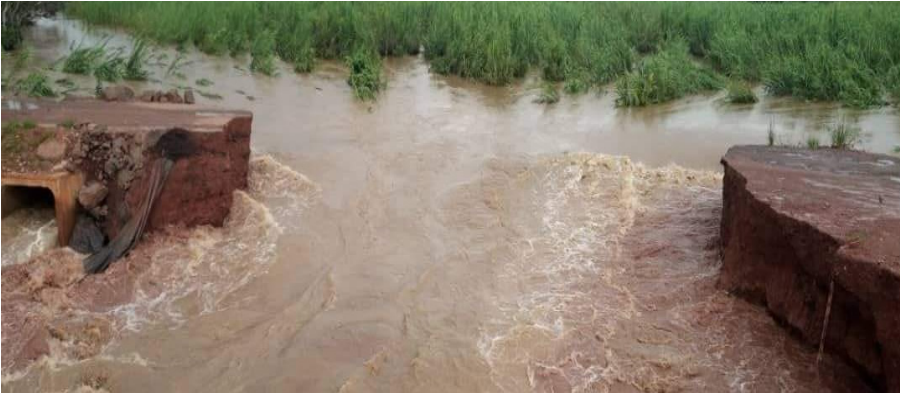
Breached Cofferd Dam in Lundazi District
