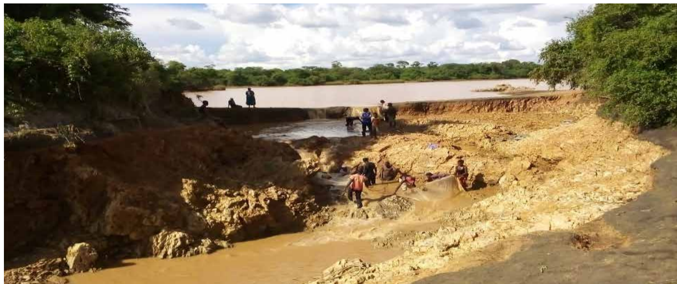
Figure 1: A picture of the Dam that collapsed at Kandesha in Central Province
